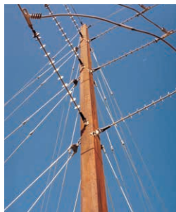
Guyed angle structures
